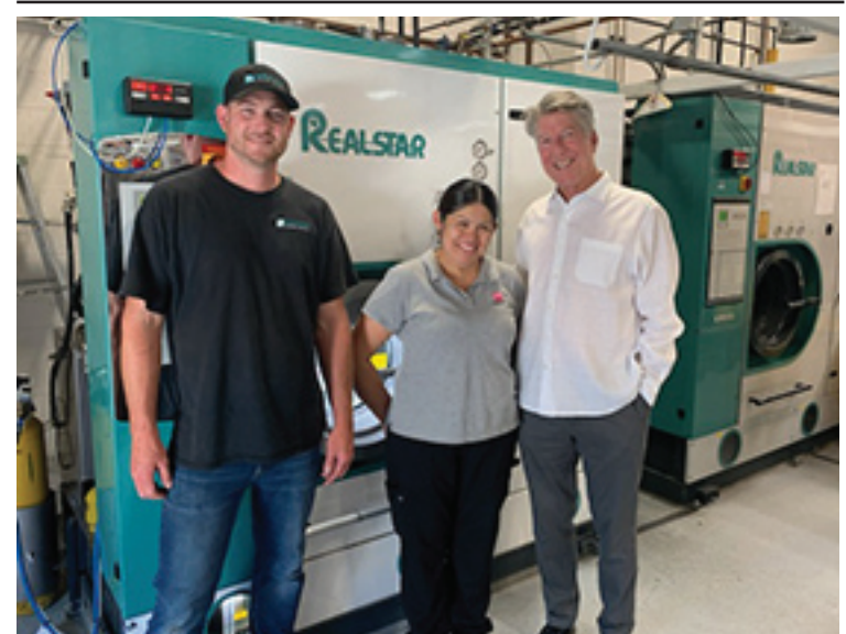
JUDI'S CLEANERS of Citrus Heights, CA, installed a new Realstar KM343 drycleaning machine, sold and installed by Abram Laundry Service. Pictured (left to right) are: Jared Abram, owner of Abram Laundry Services; Antonia Mazatzi, Judi's production leader; and Ben Combs, owner of Judi's.
